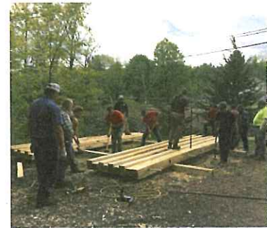
Skidder Bridge Construction workshop at the Siuslaw Model Forest. Educating landowners about the benefits of using portable skidder bridges and how to build a bridge on their property to gain access in an environmentally friendly way without disturbing water quality, as well as provide portable skidder bridges to regional loggers. Sponsored by the Watershed Agricultural Council's Forestry Program.
